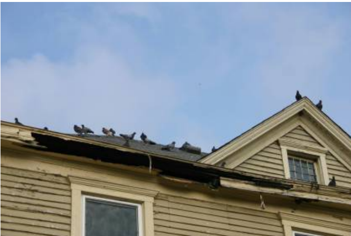
Caption: View of deterioration
